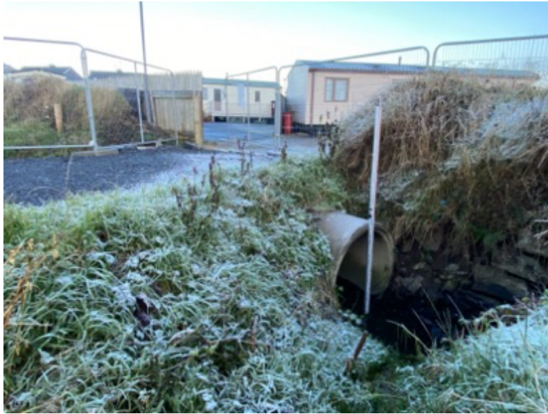
Figure 8 – Inlet to Culvert routed under Field Entrance on Western Boundary of Caravan Park
